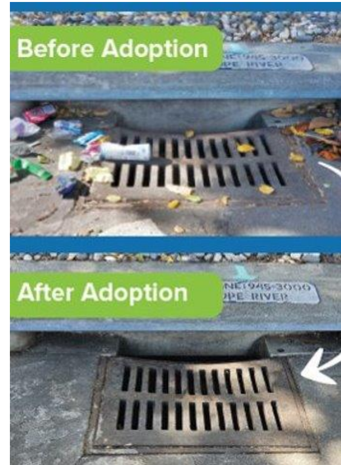
Storm drain before adoption with trash and debris strewn around it, and after adoption without trash or debris.
